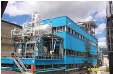
Rende –Biomass 14 MW and Solar 1 MW
